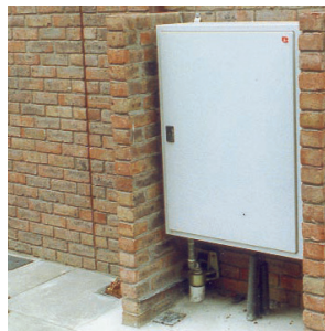
Six meter cabinet
