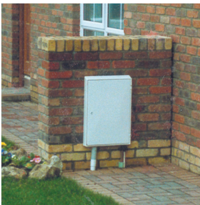
Domestic meter box
